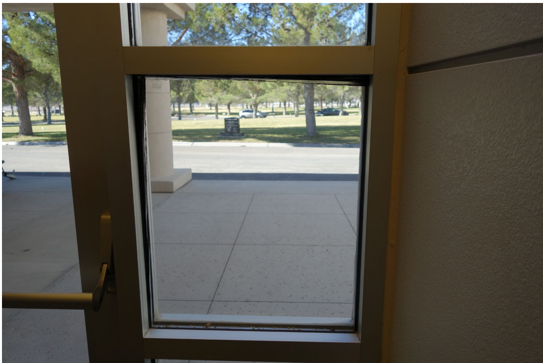
Chapel – FCA Building #2105 Description: Storefront Glazing System Repairs Needed.
