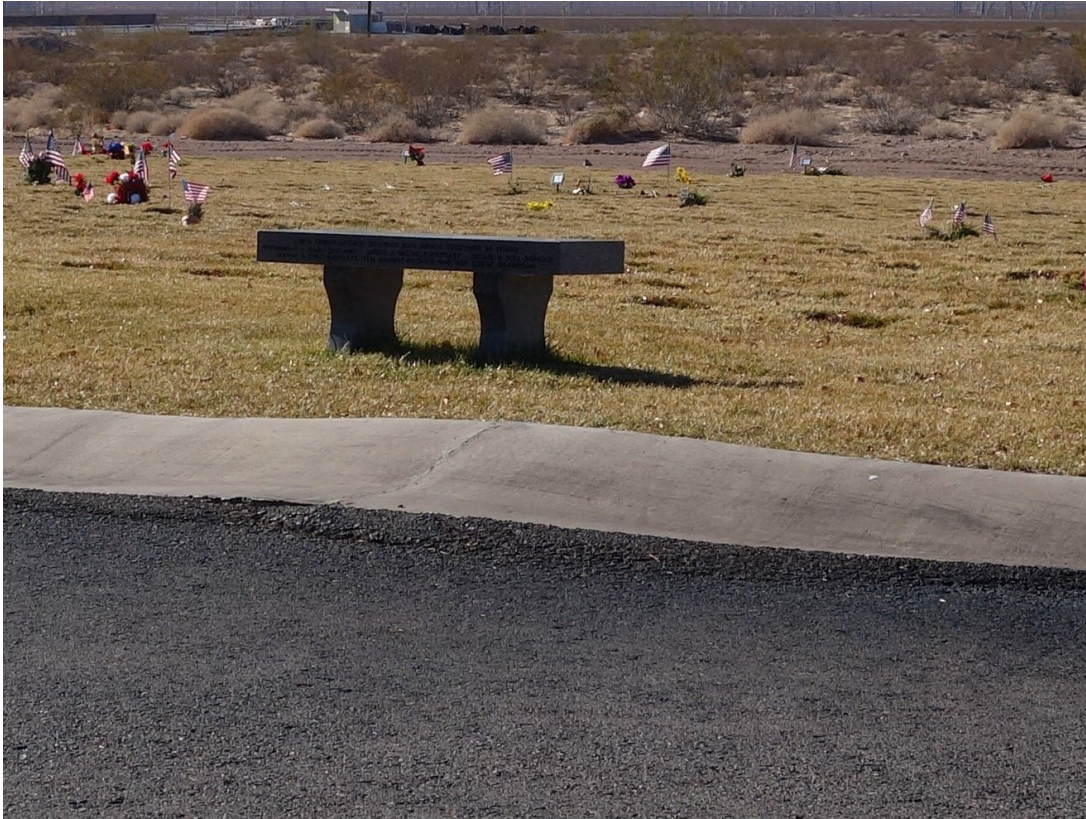
Southern Nevada Veterans Memorial Cemetery Site – FCA Site #9890 Description: Asphalt Paving Repairs.
