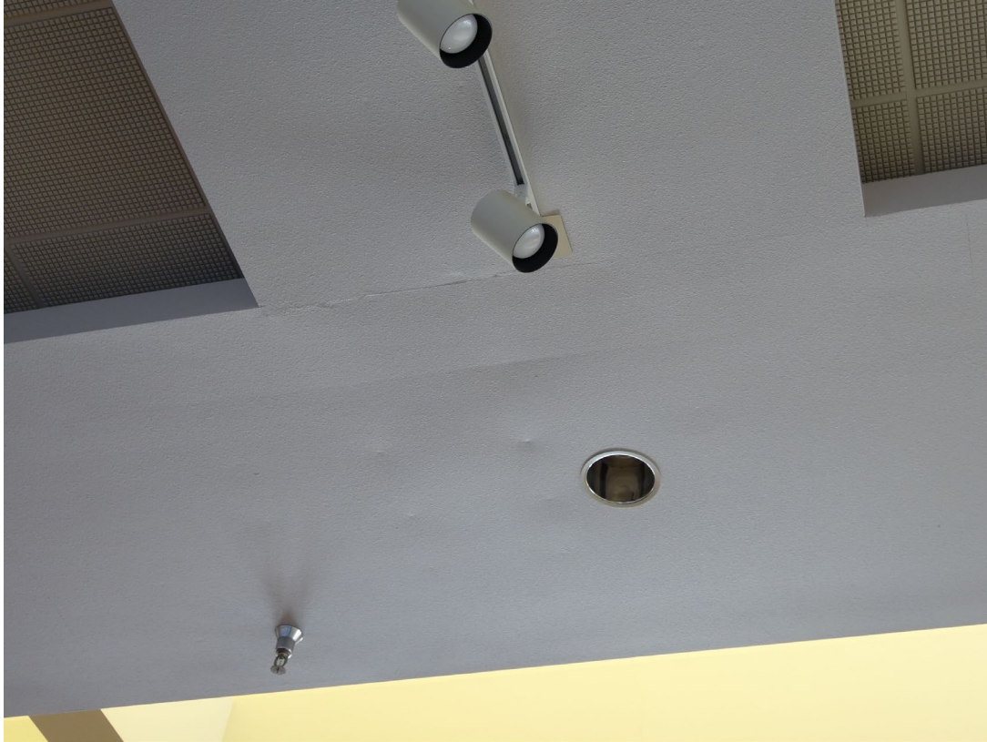
Chapel – FCA Building #2105 Description: Gypsum Board Repairs Needed.
