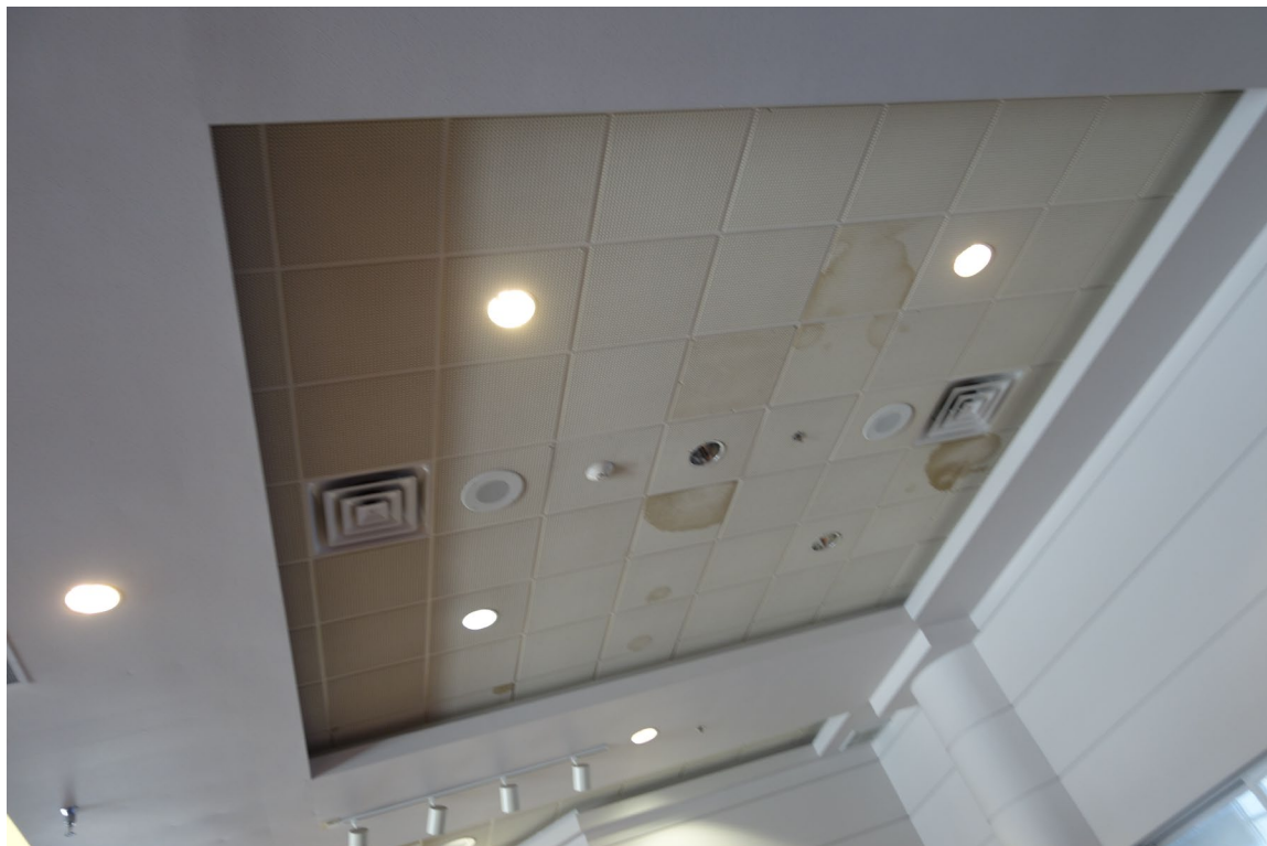
Chapel – FCA Building #2105 Description: Ceiling Tile Replacement Needed.
