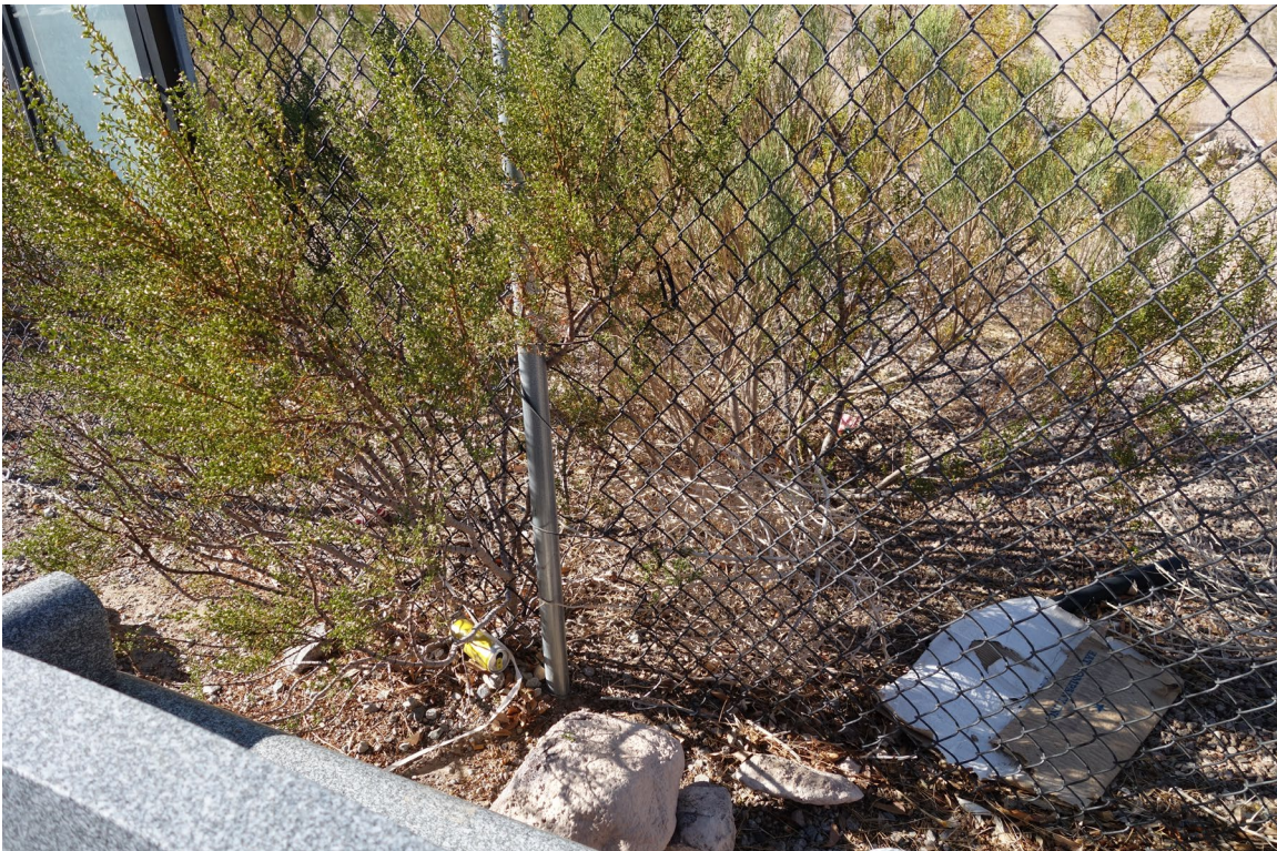
Southern Nevada Veterans Memorial Cemetery Site – FCA Site #9890 Description: Perimeter Fence Damaged During Theft Event.
