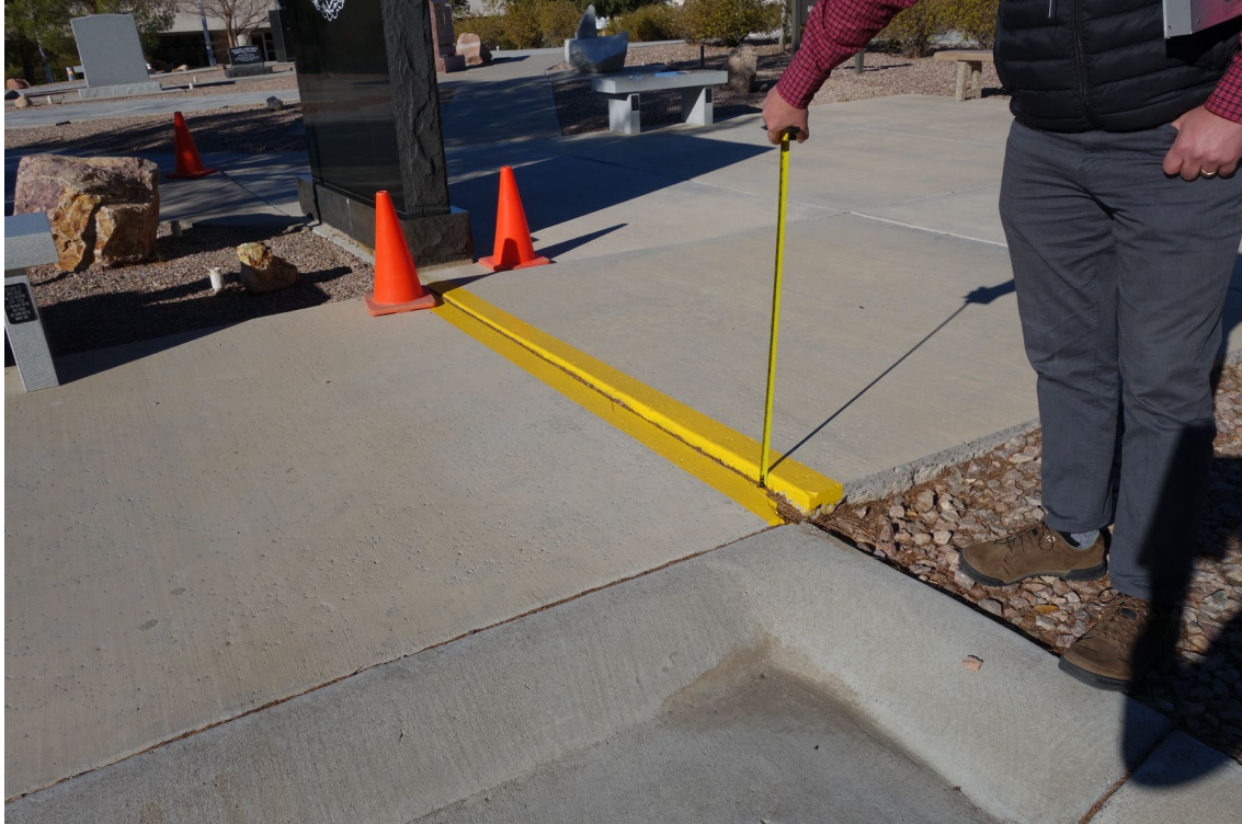
Southern Nevada Veterans Memorial Cemetery Site – FCA Site #9890 Description: Sidewalk Replacement Needed.
