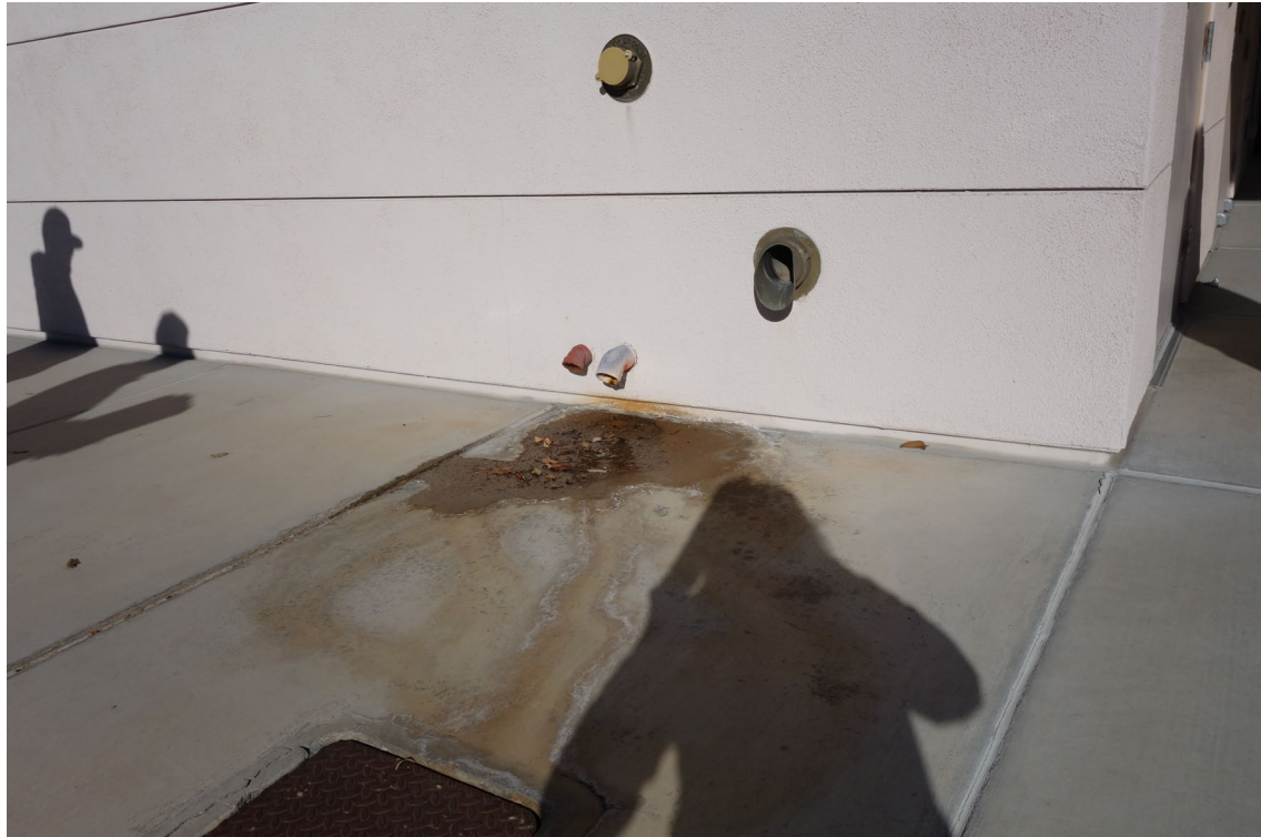
Administration Building – FCA Building #3147 Description: Drainage Modifications Needed.
